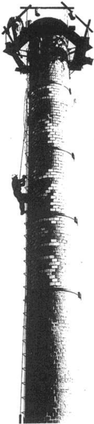
High-chimney repairman Blair Hendricks heads up the ladder to the cap (rim) of the smoke stack of the Palmer Asbestos and Rubber Corporation's plant in St. Matthews to make repairs.
